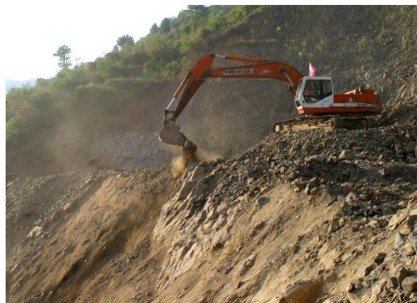
Fig. 1. Moving blasted rock to the dump to the foot of the mountain by an excavator at the KT2 construction site.
